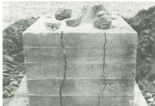
The end of the old concrete blocks on the shores around the laboratory
